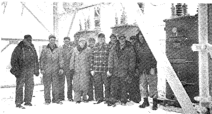
When the last of the three initial substations, the Tolstoy Substation, was energized on December 19, 1949, service was provided in all three counties, thus establishing the back bone of FEM's distribution system.
