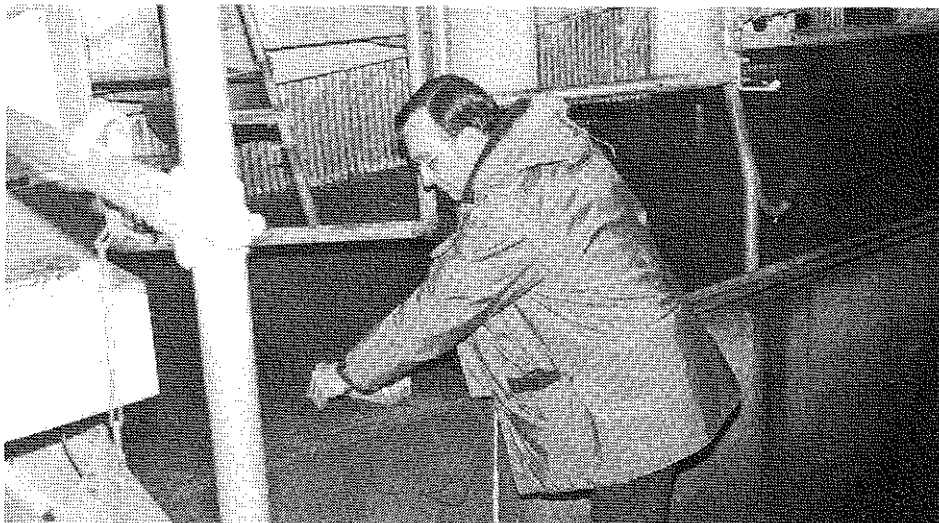
Power Use Advisor Myron Fillbach is shown checking a stanchion in a dairy facility for stray voltage.
