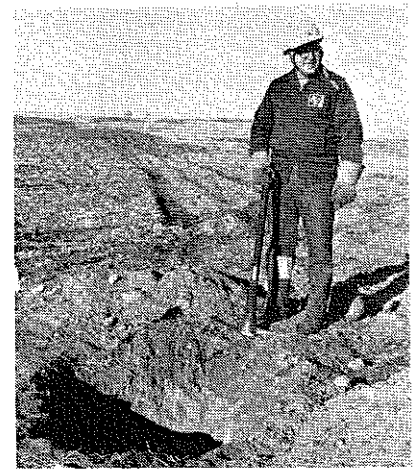
Once the fault is located, the cable must be exposed to repair the fault.
